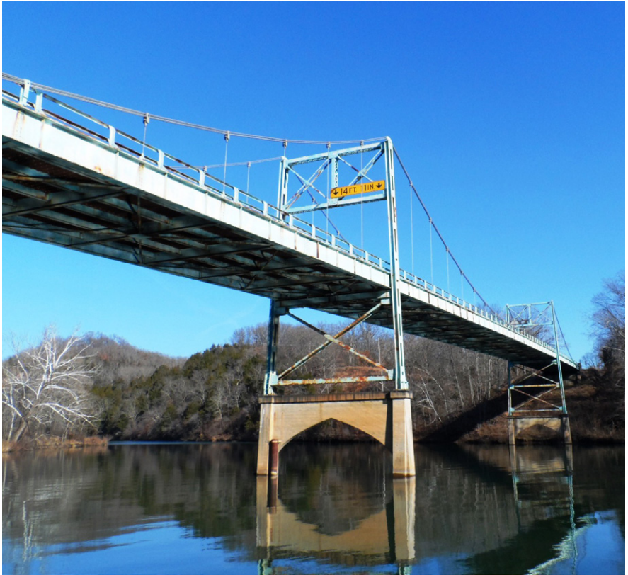
Bridge over the upper Little Niangua arm of Lake of the Ozarks in Camden County. (Bryan Vance photo)
